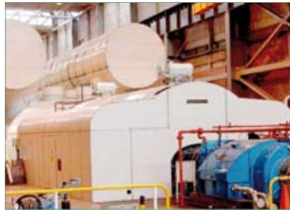
Wylfa has four turbine generators cumulatively producing 980MW.
