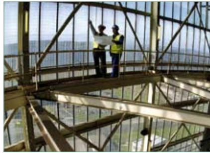
The replacement weather envelope will provide the environment necessary to demonstrate the continued safety of the reactor buildings.
