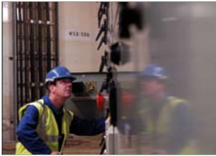
Decommissioning requires a wide range of skills and technical support in which many local firms are engaged.
