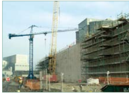
New construction is required on site to facilitate decommissioning such that the ultimate aim of final site clearance can be achieved.
